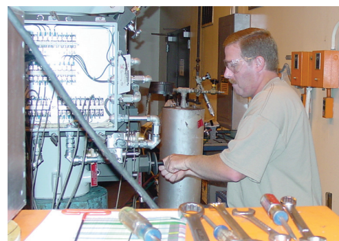
On-site mechanical service and maintenance includes 24/7/365 availability.
