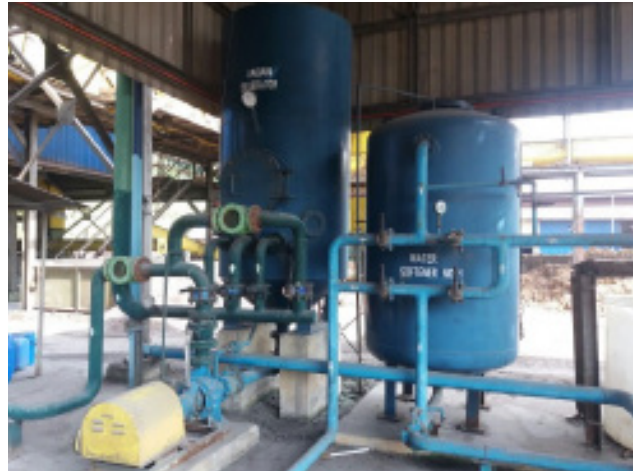
Water transfer pump (SIHI model ULNC)
