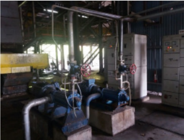
Boiler feed pump (SIHI model HEGA multistage)
