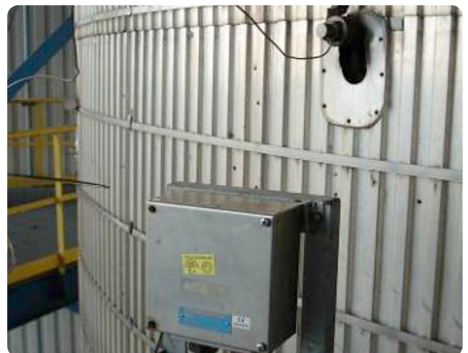
High-temperature accelerometers monitor vibrations on the coke drum wall. The resulting signals provide the operator with information regarding drum cleanliness status.
