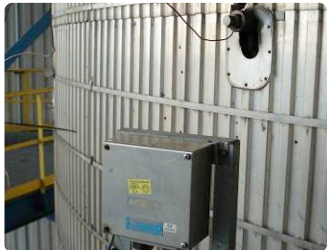
High-temperature accelerometers monitor vibrations on the coke drum wall. The resulting signals provide the operator with information regarding drum cleanliness status.
