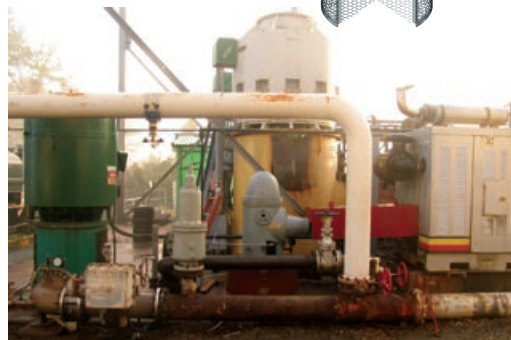
Existing vertical fire pump
