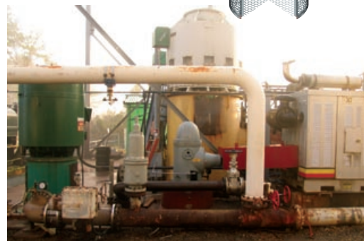
Existing vertical fire pump
